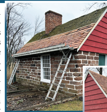
LEFT, AS THE OLD ROOF IS REMOVED, BRIGHT NEW CEDAR SHINGLES ARE INSTALLED.
